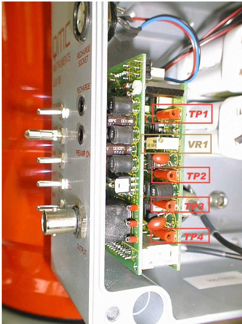
Photo 3. View of the switchboard and amplifier circuit board identifying the voltage test points and multi turn potentiometer
